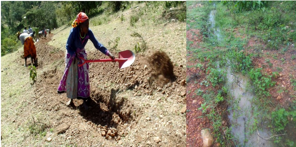
Figure 4. (a) Farmers constructing terracing in Kaporowo in 2019 and (b) the view in April 2020 on the benefits of terracing in reducing water speed, retention and increasing the time and amount of water infiltrated. (Photograph taken by Mr. Alkamoi Bonface, University of Eldoret)
